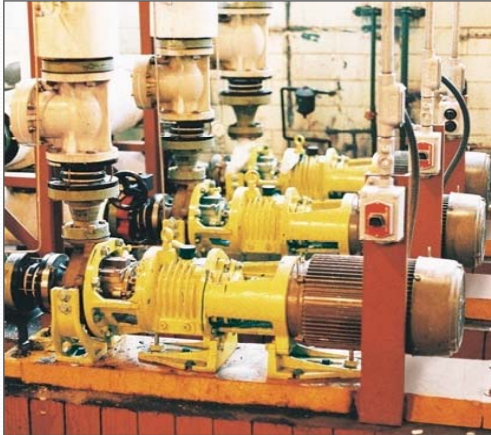
A Pumping System in an Industry.
